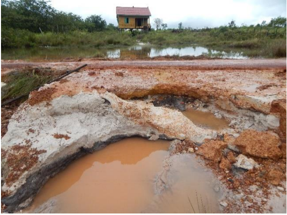
Photo 3.5. Road condition in the relocation site during the monsoon season Source: Author
